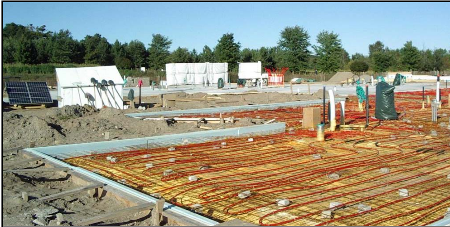
This photo, taken in September, clearly shows some of the 17,000 feet of polyethylene pipe for the ground source heat system placed in the floor slab. In the background to the left can be seen the solar panel used to provide power to the work site, and in the far centre are stacked some SIPs panels for the walls.
